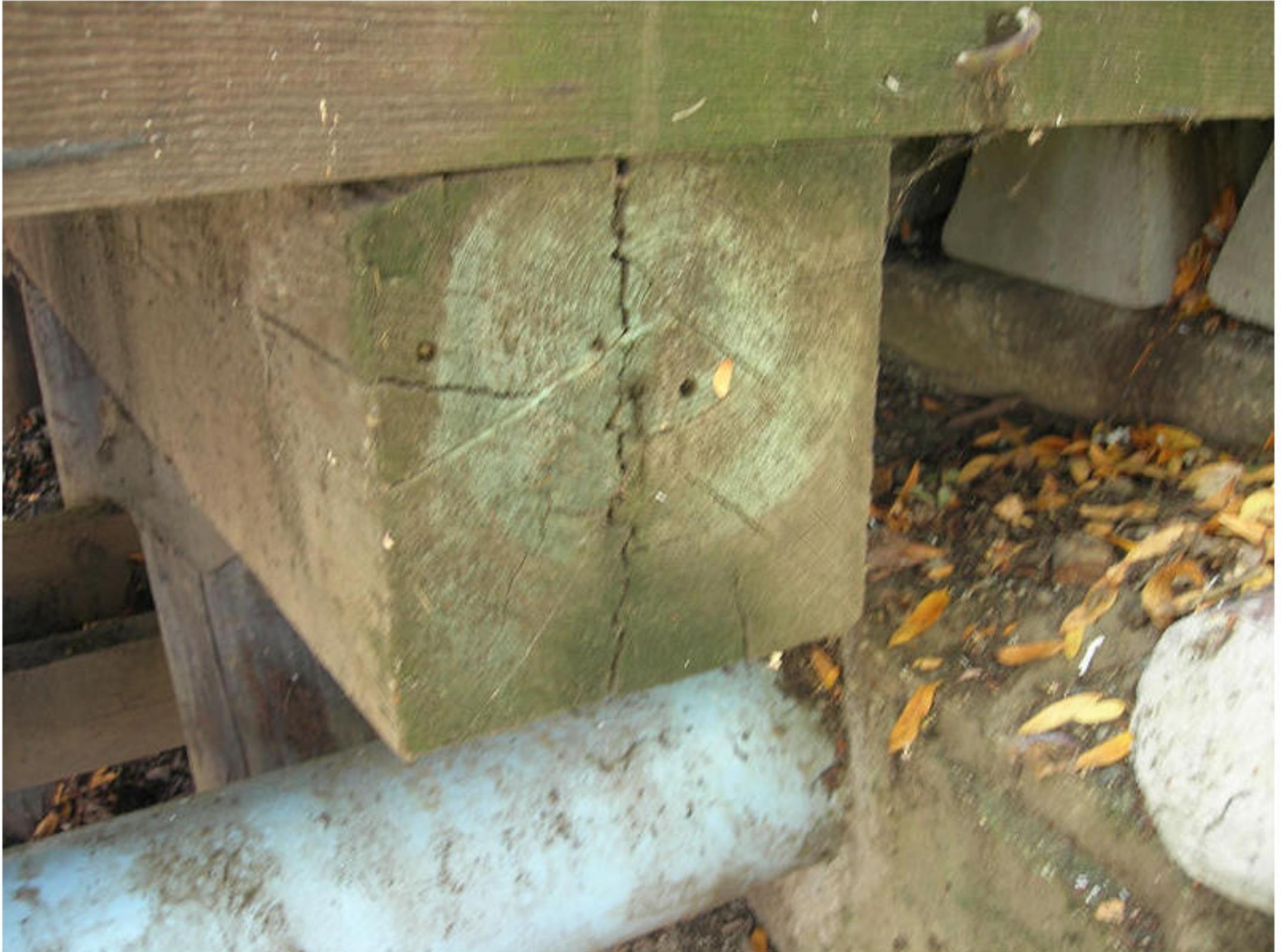
Photo No. 1 Split on Bent cap 2 left.
