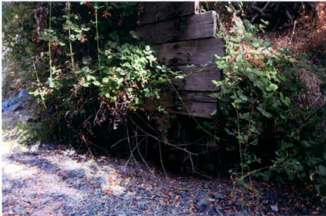
Scour of the timber wall downstream of the bridge
