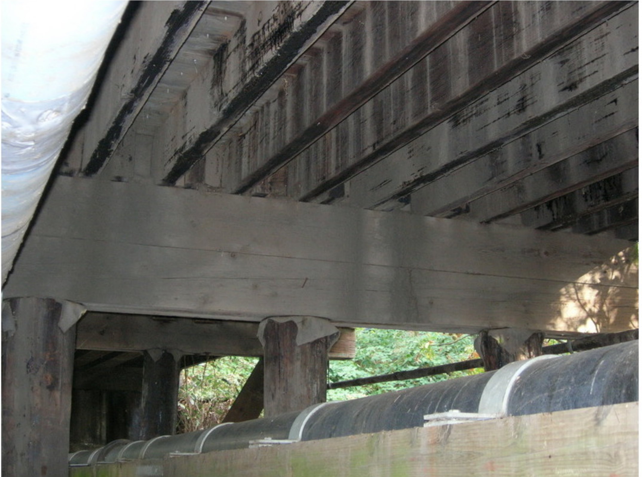
Photo No. 6 Bent cap 4 has a horizontal check full length.
