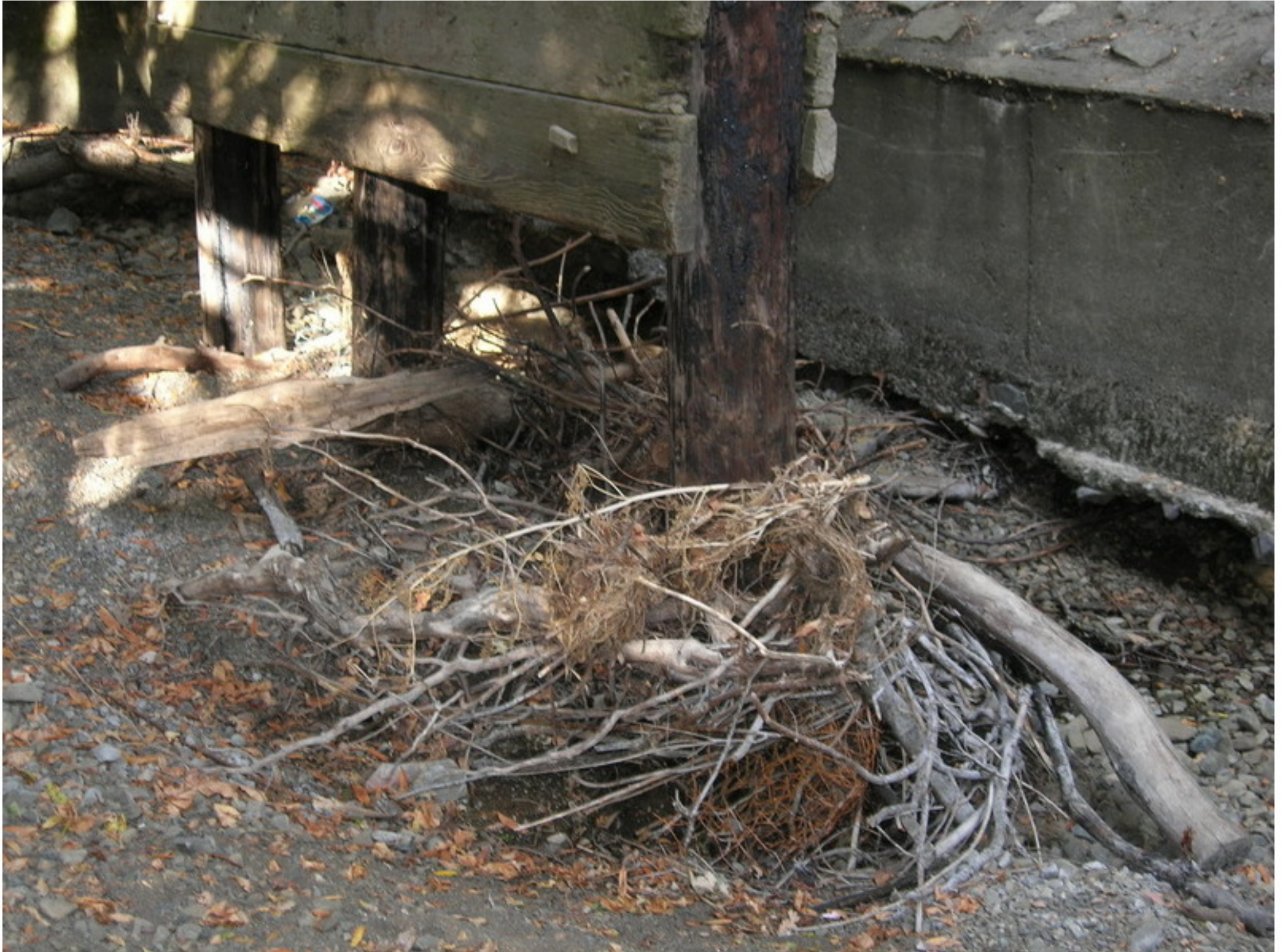
Photo No. 5 Debris at Pier 4.
