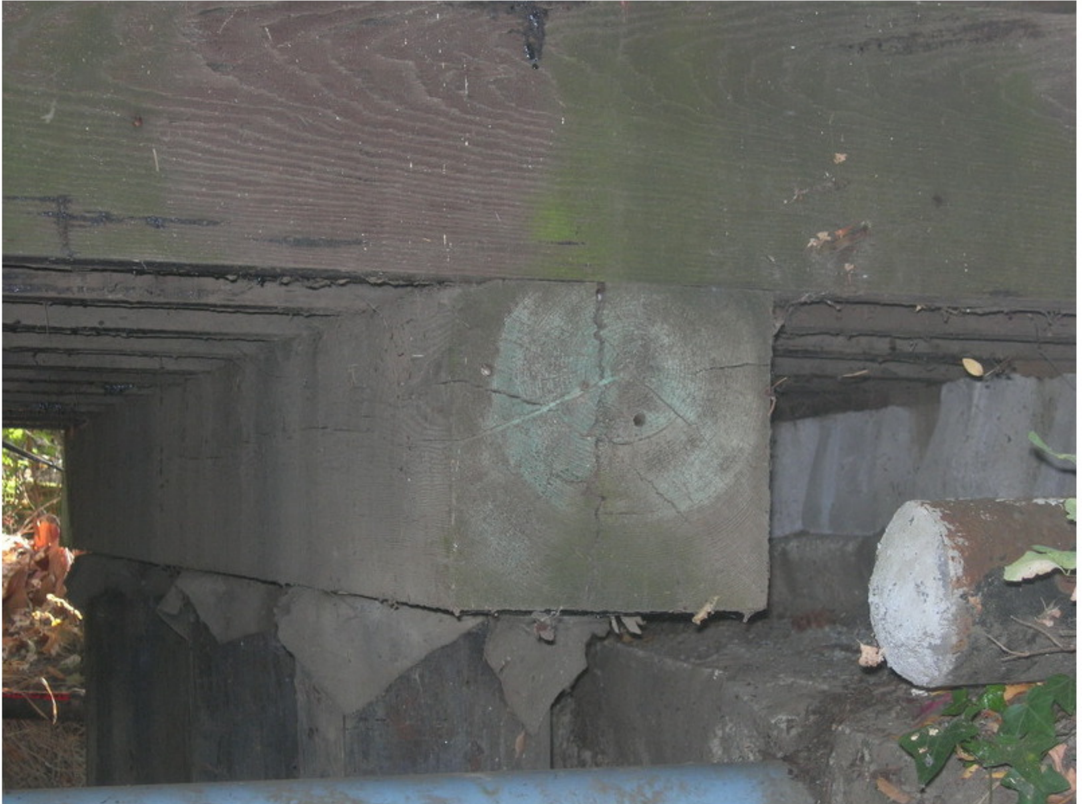
Photo No. 7 Vertical split in Bent cap 2.
