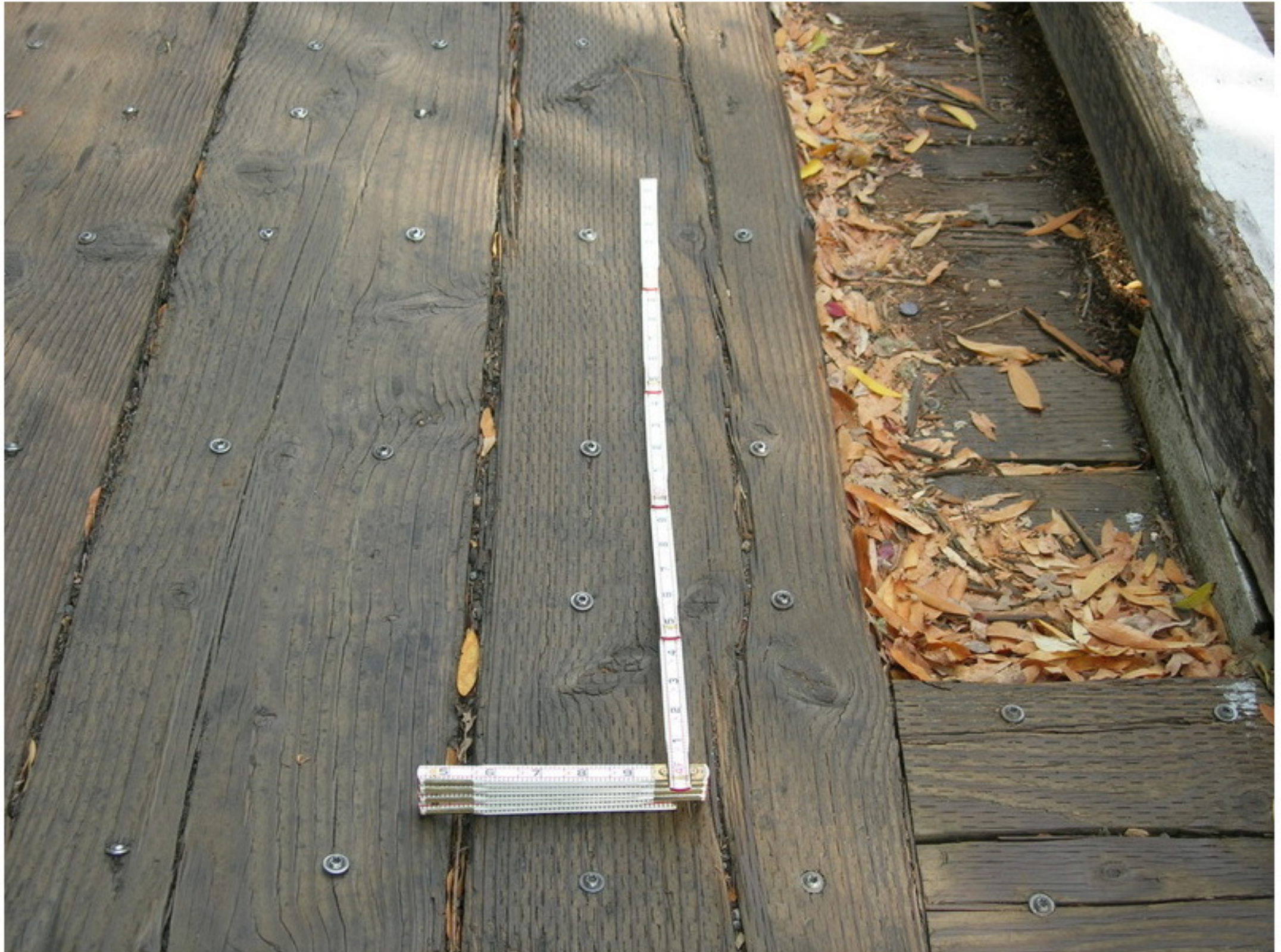
Photo No. 3 Deck runner planks split.
