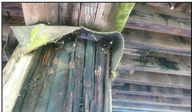
Split Pile Head at Pier 3
